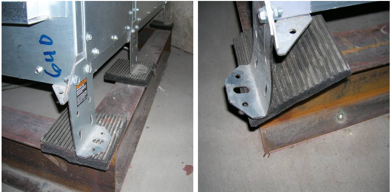
Figure 4: AHU mounting feet not anchored to floor mounts.
